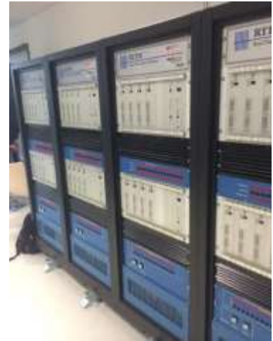
Figure 10. Eight racks of RTDS in ACS-Lab RWTH Aachen University where P3.4 student Moein Manbachi is on exchange. Each rack supports around 22 electrical nodes.
